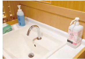
Installation of alcohol-based disinfectants
